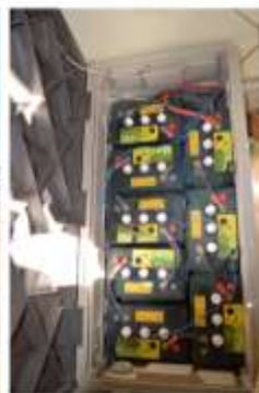
Each EMFES unit stores electricity in eight lead acid batteries
